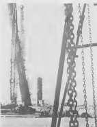
BREATHAKING moment was the rising of the 130-foot-long pipe still over that tips the scales at 180 tons. UN MOMENTO di suspeso tabata himento di e toron aki di 130 pia largo a e Pipe Still. E ta pisa 180 ton.
